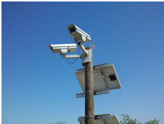
One or more cameras on AC or Solar Power
